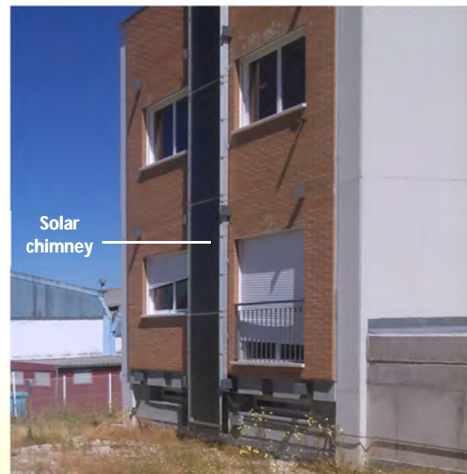
Solar chimney in EDEA demonstrators.
