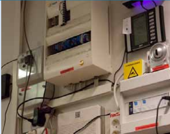
Monitoring equipment in smart housing
