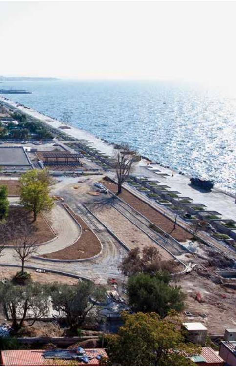
▶ Rehabilitation of the seafront at Thessaloniki, the second largest city in Greece.
