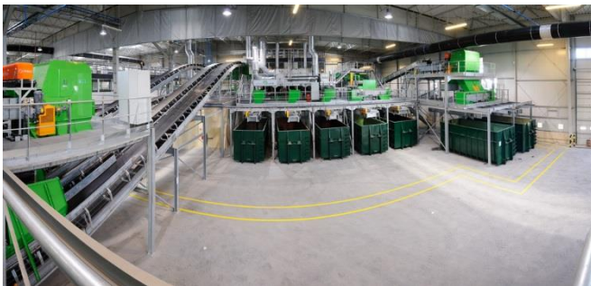
Figure 3. Photos of the sorting plant
