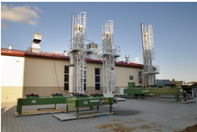
Figure 1. Photos of the biogas power facility
