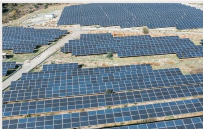
Solar Energy Power Plant
