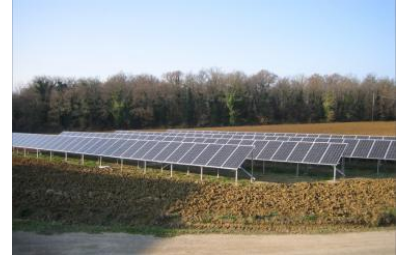
Torre Colombaia – photovoltaic panels
