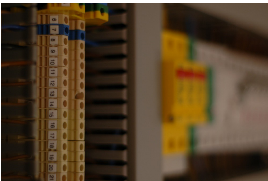
Fig. 81: correctly marked terminals in the distribution box
