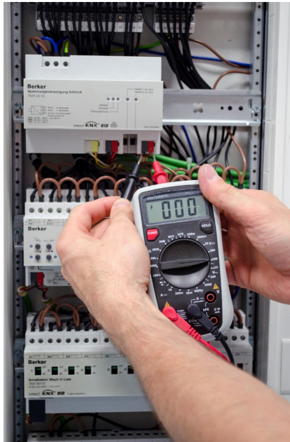
Fig. 82: BUS voltage measurement on KNX device
