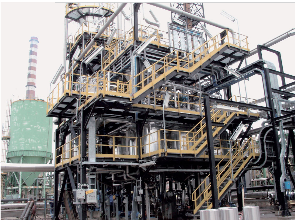
LIFE demonstrates the relevance of emerging or insufficiently developed techniques. The picture shows the new regeneration unit of the Sanazzaro refinery (p. 22).
