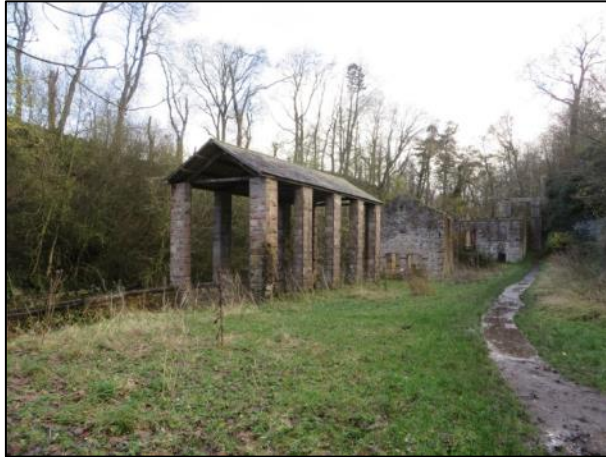
This photo shows the maintenance of weatherproof traditional farm buildings under option ED1. This feature was assessed as having a 'conserving' effect on landscape.
