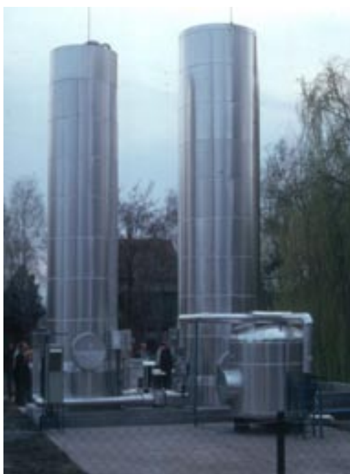
Storage tanks in the Kistelek geothermal system, Hungary
