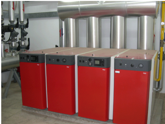
Figure 8-3: Boiler of the Municipal Swimmingpool in Abrantes.
