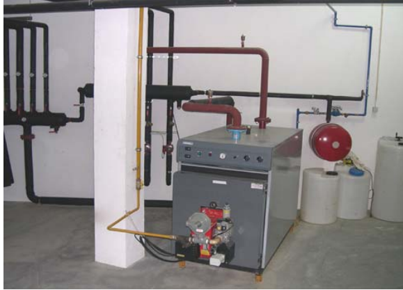
Figure 8-2: Boiler of the Municipal Swimmingpool in Marvão.
