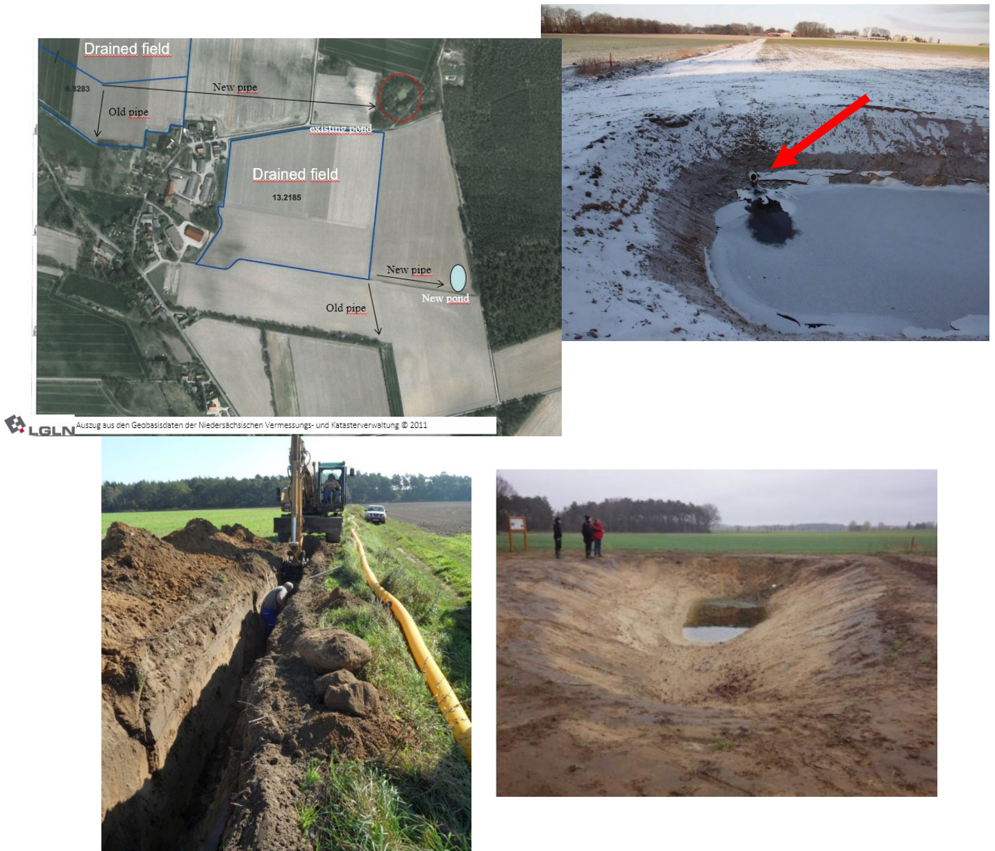
Figure 6: Construction of alternative collection drain before leading into a creek and now leading into a newly created seepage pond (see red arrow) in 2010/11. The pond meanwhile is completely hidden by shrubs and young trees. Pictures by J. Martens, Waterboard Uelzen
