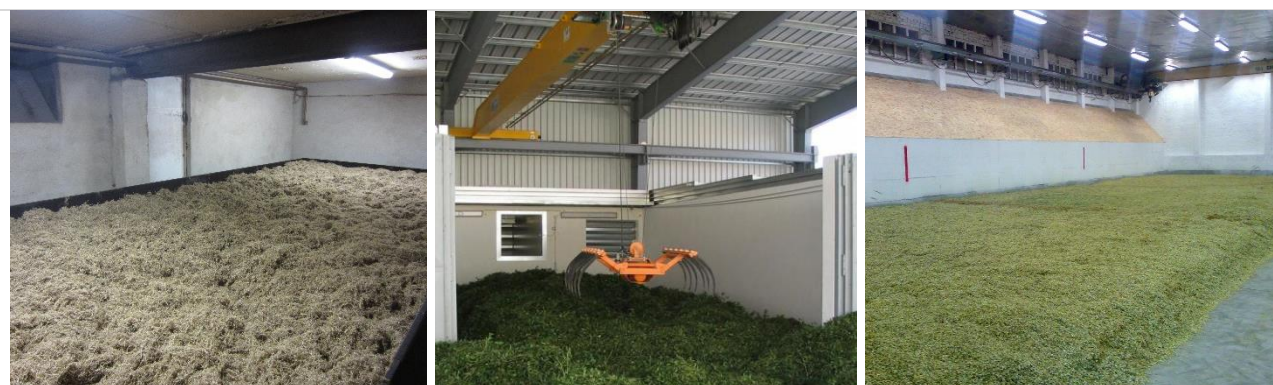
Figure 2. Flat-bed drying of herbs (Source: Left to right- Argyropoulos/UCD, Ziegler/ATB, Planungsgruppe Fölsche)
