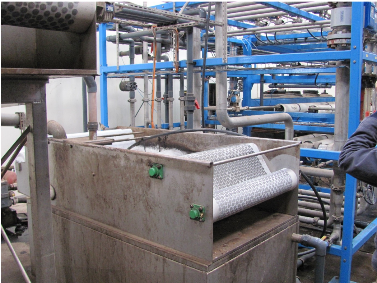
Figure 5. Ultrafiltration plant used for pig slurry treatment
