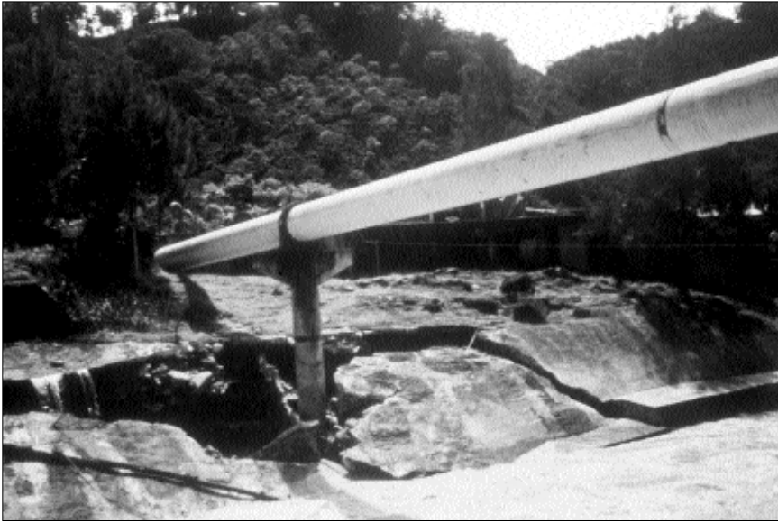
Flood damage to the bridge supporting the main water pipe of the Orosi system in Costa Rica in October 1999. Some 500 tons of concrete were displaced.
