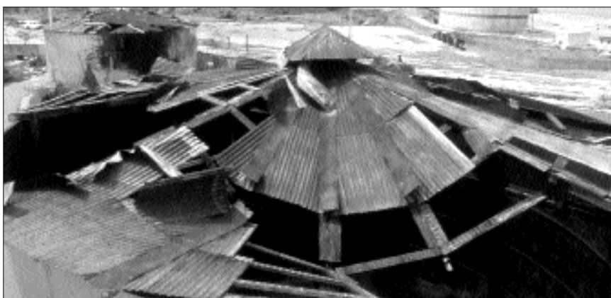
Damage to the roof of a water tank sustained during a hurricane.
