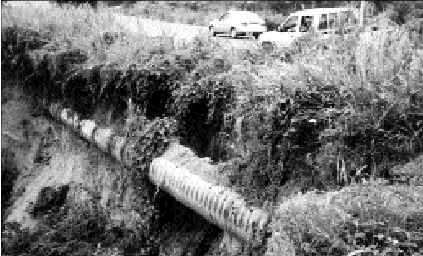
Preventive measures reduce the vulnerability of systems. Exposed piping in Ecuador.
