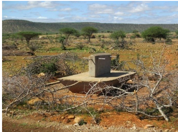
Picture 8: Water point for host community awaiting for completion of the system
