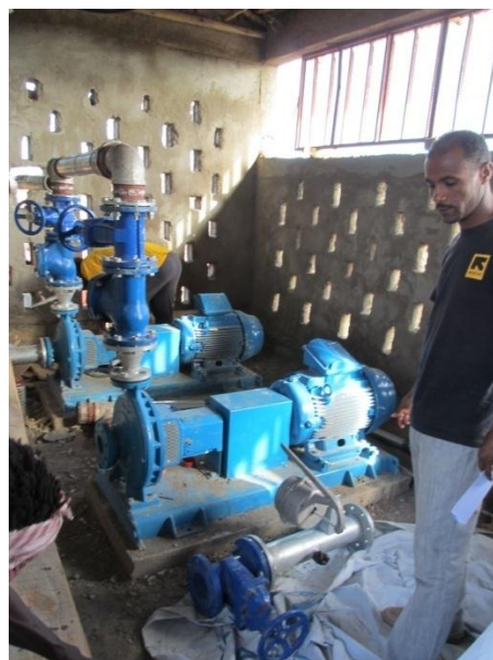
Picture 15: Boosting station
