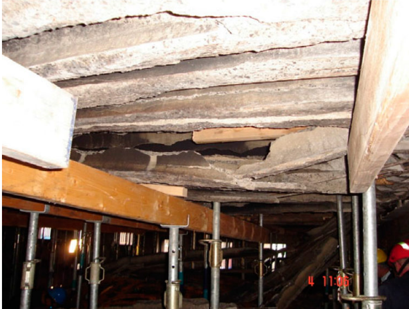
Fig. 5: Damage occurring in the car park fire at Lloydstraat Rotterdam (Fig. 25 from DE FEJTER/BREUNESSE [4])
