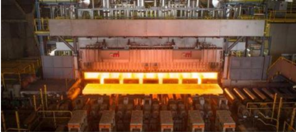
Figure 4 – Slab reheat furnace
