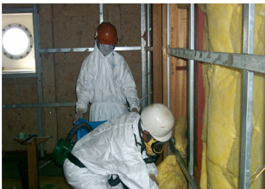
Chinese workers, equipped with protective clothing and personal equipment, removing insulation material as part of pre-cleaning (courtesy of T. Blankestijn, P&O Nedlloyd)
