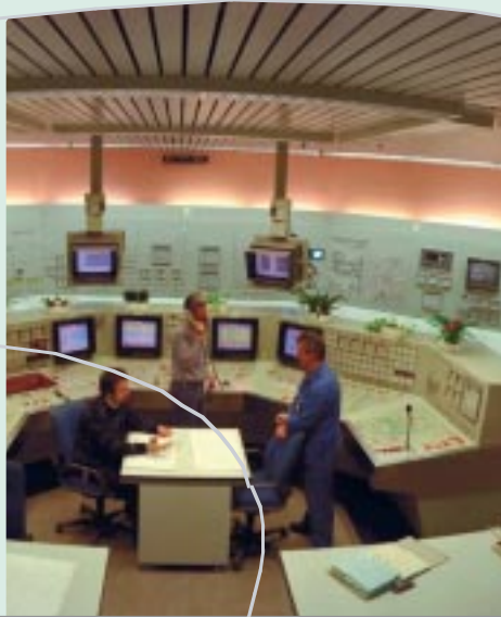
A nuclear power plant control room
