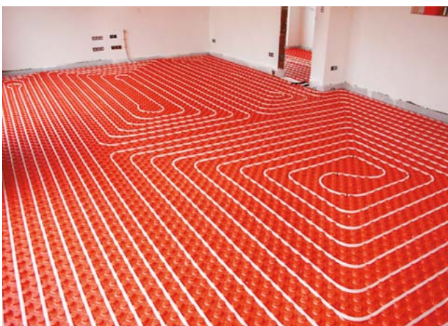
Photograph 2.2: Built-in electric system
