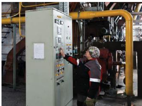
Gas installation in the boiler house at Molodohvardiysk coalmine, Luganska oblast
