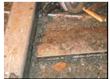
Detail of split in moveable deck
