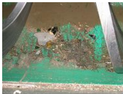
Detail of wear on a screw casing
