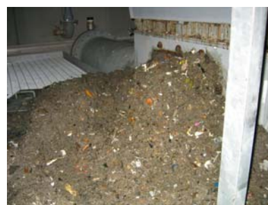
Digester feed screw blockage
