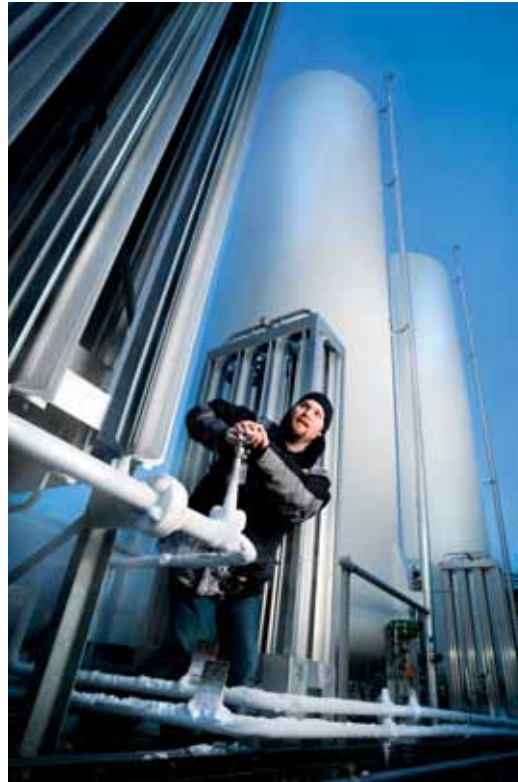
A biogas production plant in Henriksdalsverket: one of Stockholm Water Company's waste-water-treatment plants.
