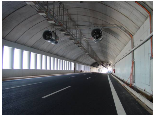
ELECTROMECHANICAL INSTALLATIONS ATTIKI ODOS HIGHWAY
