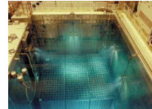
Used fuel storage pond
