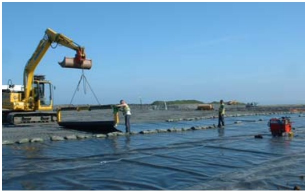
Gas collection liner.
