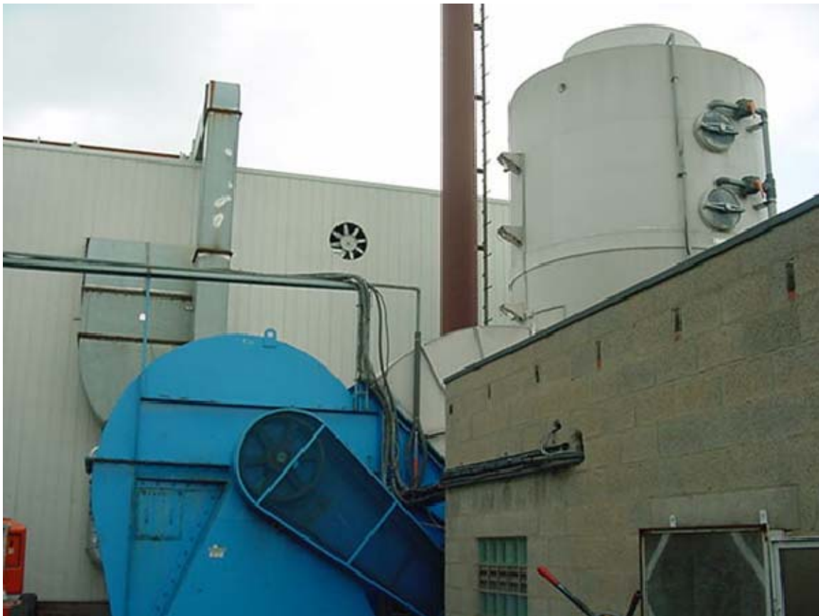
Fumes washing tower Unit 1
