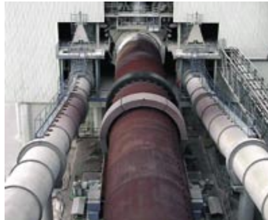
Rotary kiln with tertiary air ducts
