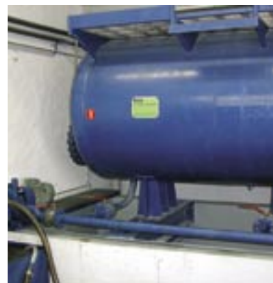
Collecting old oil for disposal
