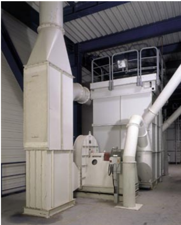
Silencer on a filter system
