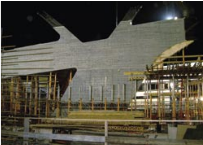
The central building of the new BMW works in Leipzig, constructed to the design of the architect Zaha Hadid using Aaton Ultra self-compacting concrete on the basis of our CEM II/B-S 32,5 R.
