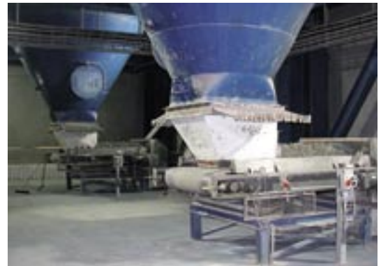
Limestone supply hoppers
