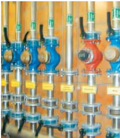
Cold water distributor
