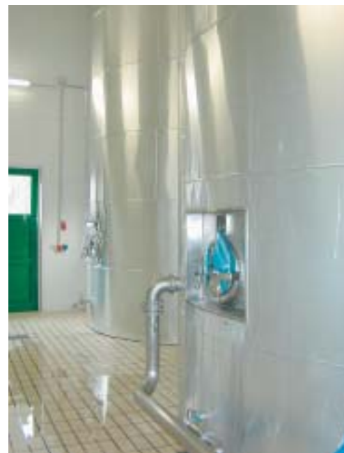
Tanks for cold and hot water
