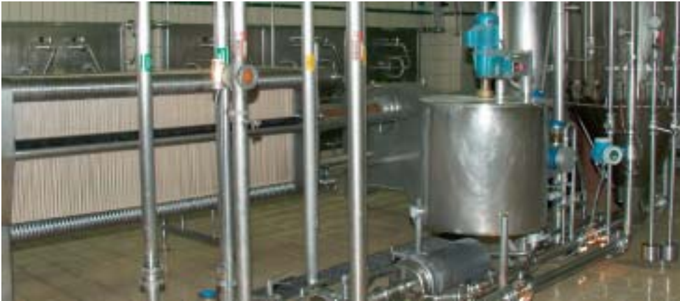
Careful work going on in the filter cellar
