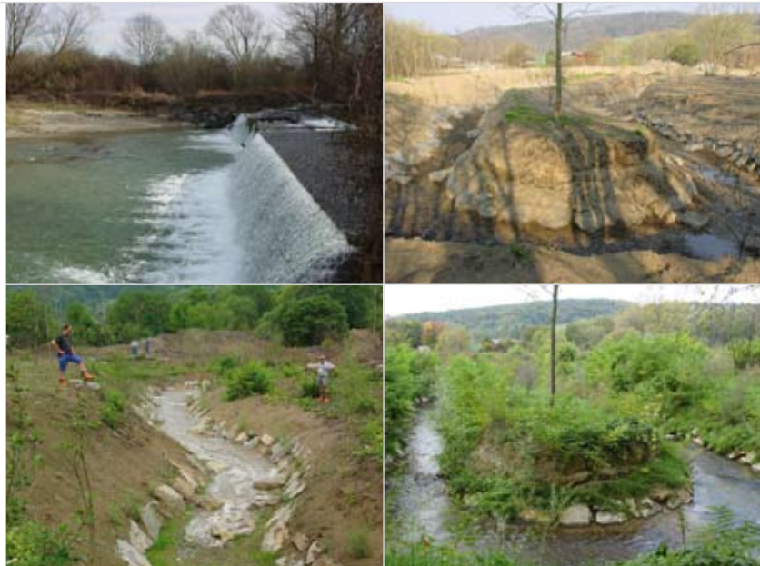
LIFE project work – top (left to right): opening a new side channel that allows for the migration for fish at the weir 'Eibelsau' – weir, and construction of the side channel – below (left to right) first water flowing into the new channel, and channel with flowing water and vegetation allowing the fish to migrate upstream
