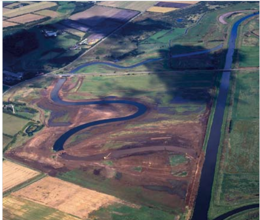
Aerial view showing the former straightened river section (right) and the re-meandered section during the construction period (left)
