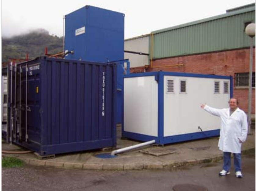
A horizontal transport container houses the hydrolysis tank, the heating system, the control panel, two pumps and a macerator.
