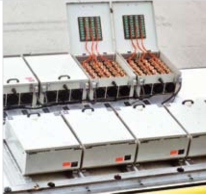
Close-up of ultracapacitors.
