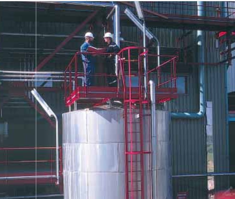
Solvents recycling: Speichim Processing.
