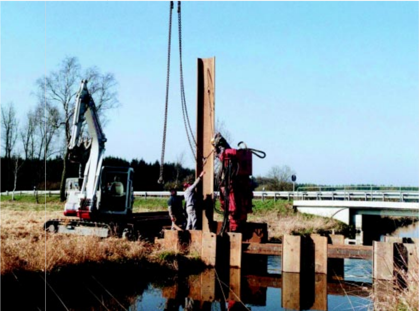
Building a dam across the Kanzach stream to raise water levels. (LIFE project "Federsee"). Photo © Jost Einstein
