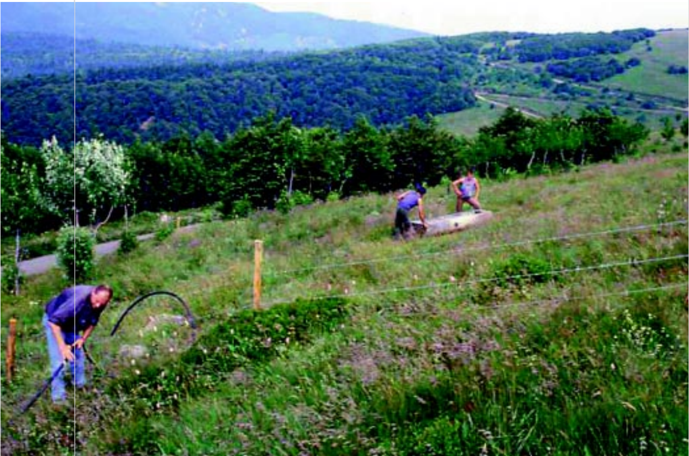
Installing a drinking trough for livestock (Alsace, LIFE project "Pelouses sèches"). Photo © Bernard Destrieux, CSA
