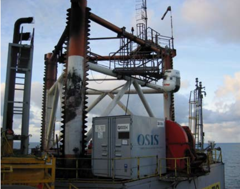
OSIS sensor system shown here at the front of the oil rig.
