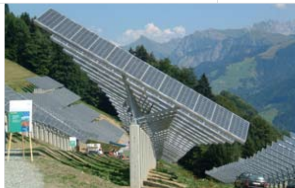
PV (Photovoltaic) panels: helping to achieve e2 (energy audit status).
