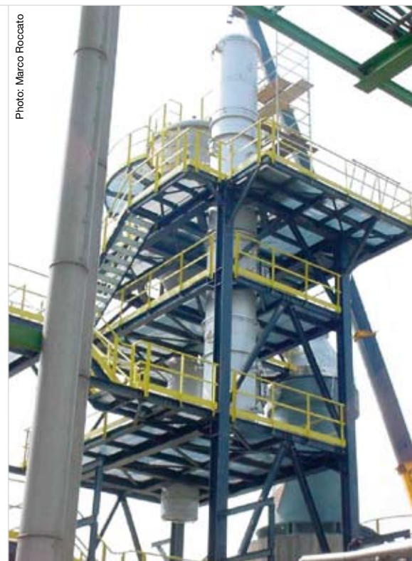
Details of the new plant showing the stripper (top) and evaporator (bottom right).
