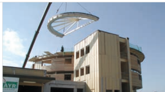
The entire wooden structure and the building's cladding were prefabricated in a workshop and assembled in only nine days.
