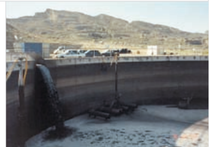
Biological reactor for continuous treatment of the wastewater.
