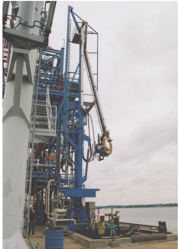
Figure 9 - Loading arms with vapour return facility
