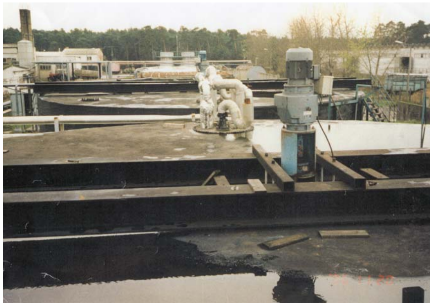
Photo 1: Top view of the biogas reactors
