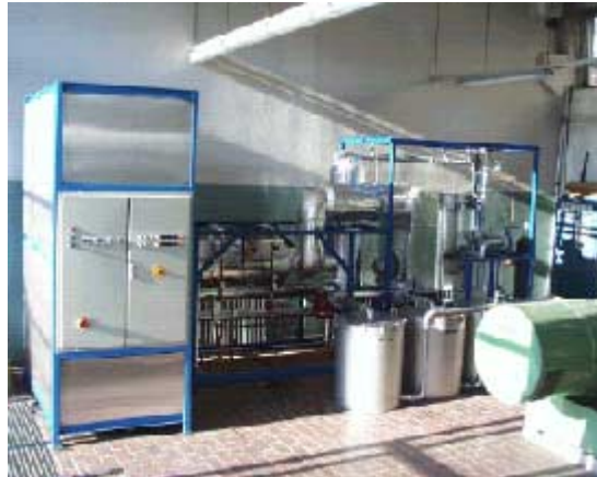
Fig. 29 Gas processing unit of Rodenkirchen WWTP
