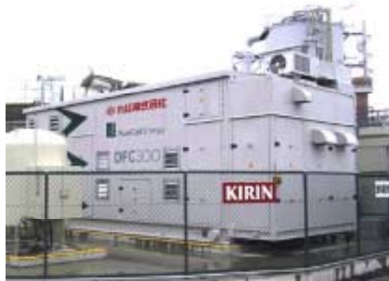
Fig. 31 250kW fuel cell operating on brewery ADG
