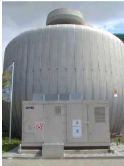
Fig. 28 PC25C fuel cell in Rodenkirchen WWTP
