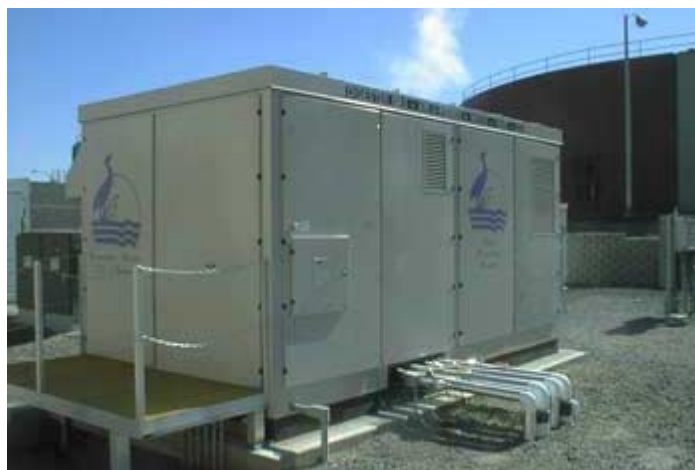
Fig. 49 The Portland facility operated on ADG from a wastewater treatment plant [UTC Fuel Cells web site]
