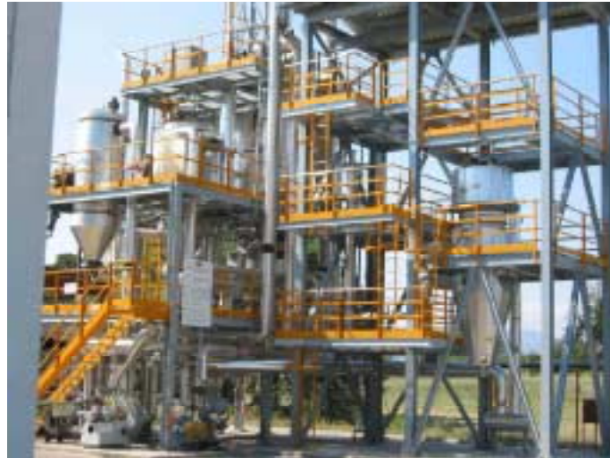
Fig. 27 Ansaldo Fuel Cells MCFC pilot plant
