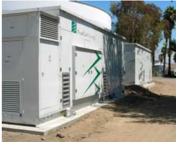
Fig. 37 A 500kW installation at El Estero waste water treatment plant, Santa Barbara, CA [FuelCell Energy web site]
