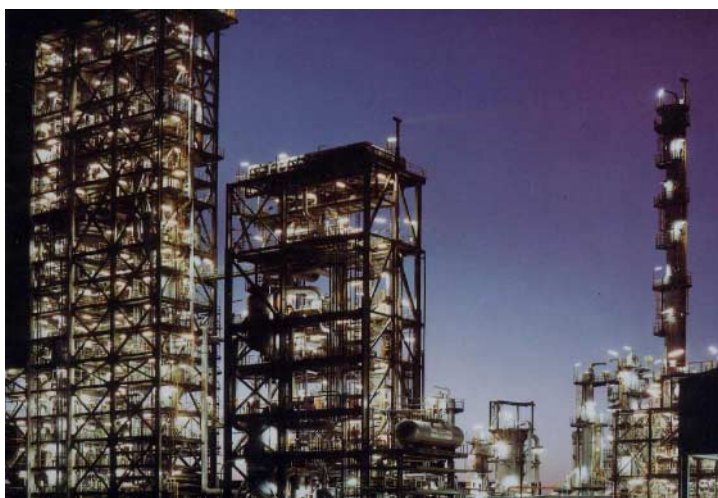
Figure 5. Rheinbraun AG's Berrenrath site, Germany. HTW gasification technology has been used to co-gasify brown coal, sewage sludge and scrap plastics.
