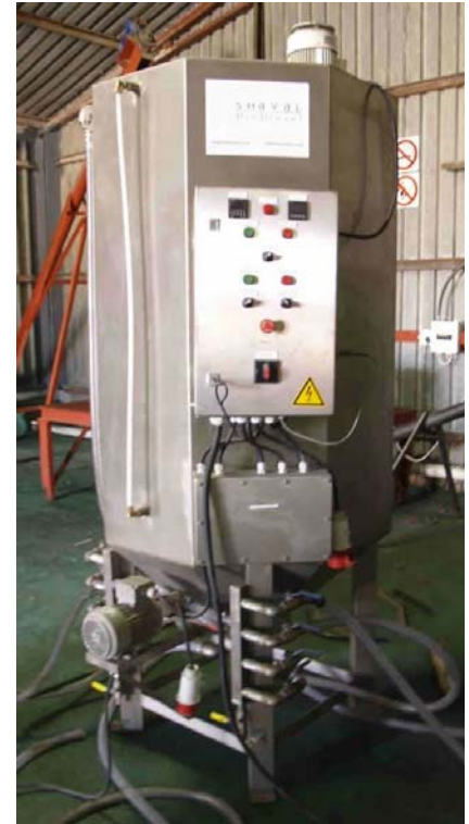
Shaval Biodiesel: Transestification takes place in a 1400 litre vessel constructed from stainless steel
