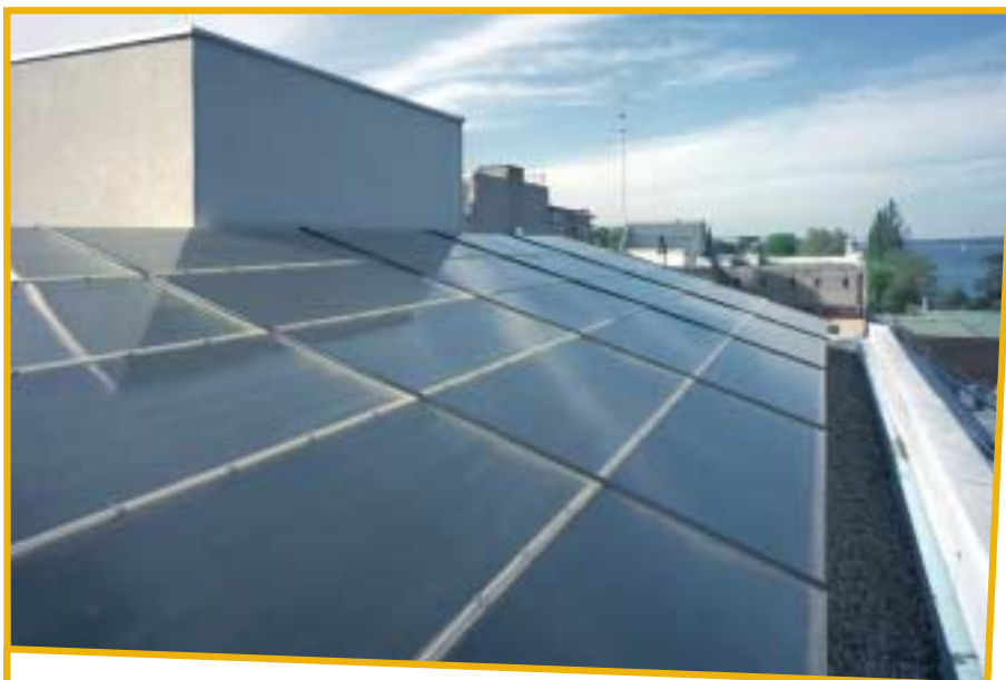
Solar thermal installation in the city of Geneva
