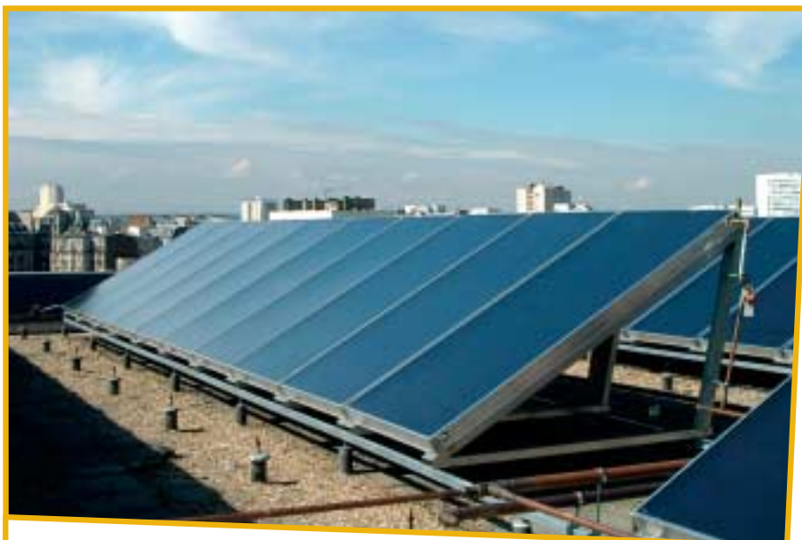
Detail of solar panels, installed on a roof
