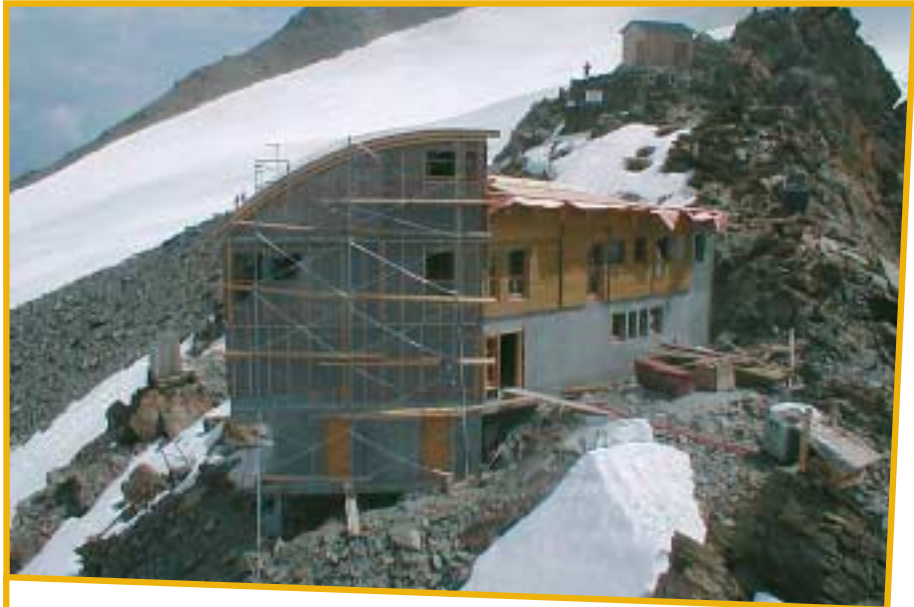
Detail of a mountain hut equipped with RE supply systems
