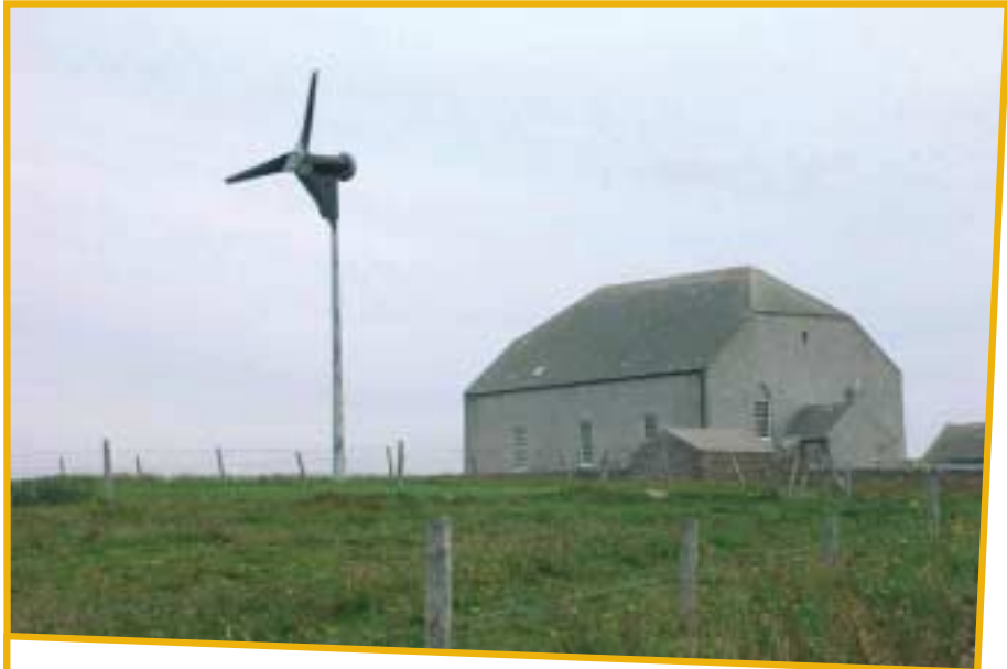
Wind turbine generator in an isolated area
