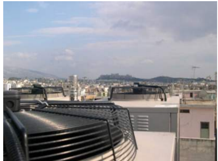
Hotel Oscar – Athens, Greece. 423 kW heating/ 220 kW cooling
