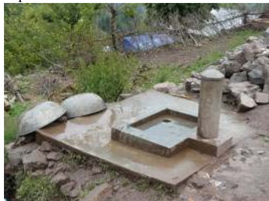
Figure 15: This good quality ECHO-funded standpost is likely to provide water for many years.
