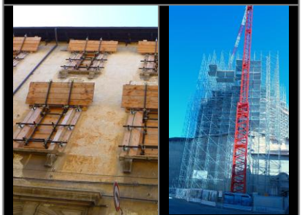
L'Aquila city center is currently held up entirely by scaffolding (10/2011)
