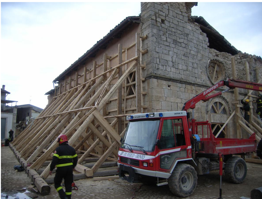
Figure 6: Sheltering of the Cathedral of Onna
