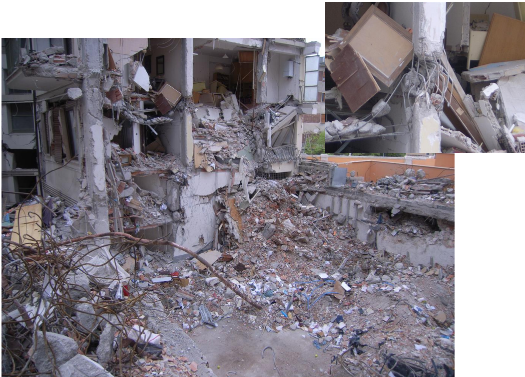
Figure 9: Collapse of old reinforced concrete building
