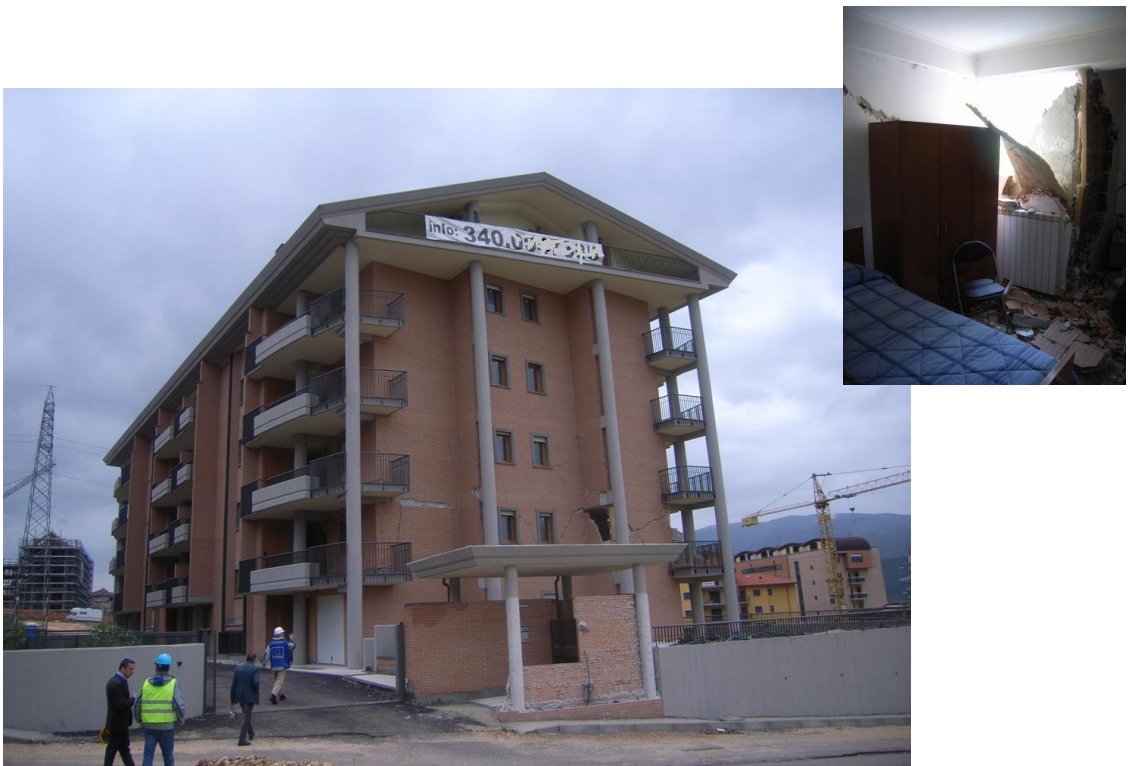
Figure 10: Very recent building which suffered extensive nonstructural damage
