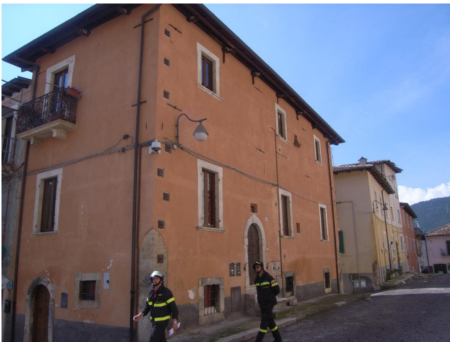
Figure 8: Historical centre of L'Aquila: apparent good performance of old masonry building strengthened with ties
