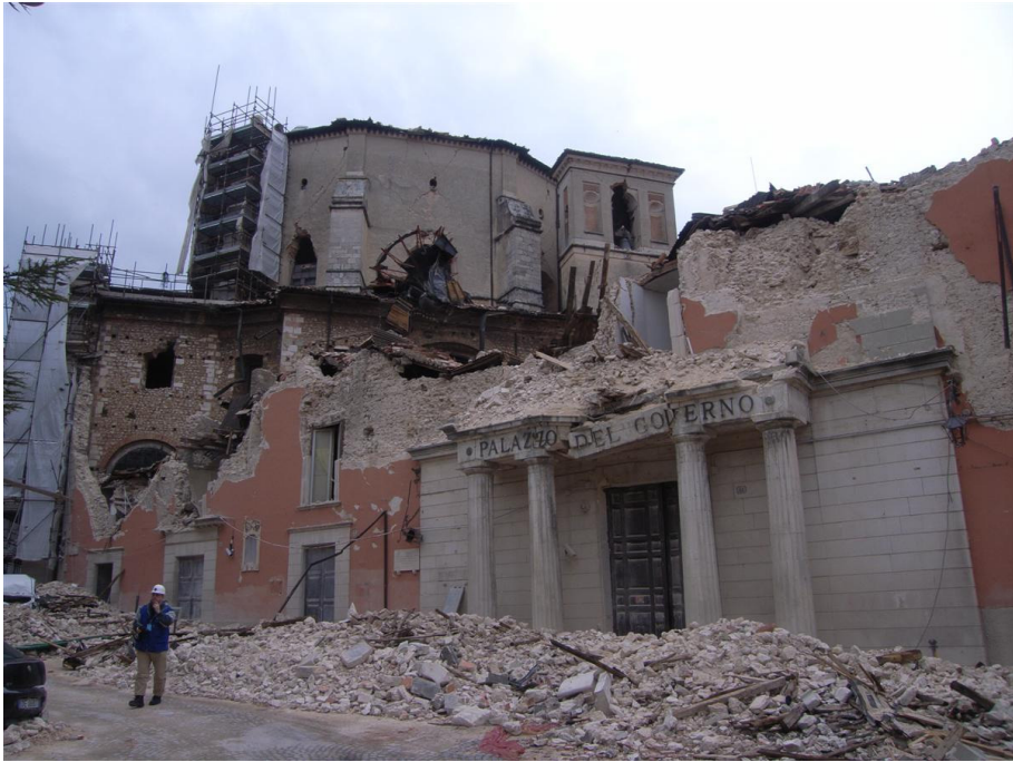
Figure 1: Damage to the Prefecture building.
