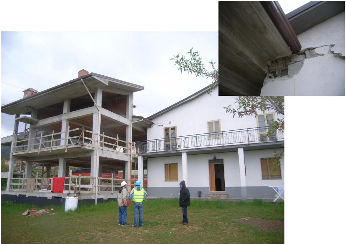
Figure 11: Consequences of the lack of seismic separation joint
