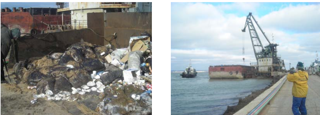
Figure 10 – a) and b) temporary storage barge
