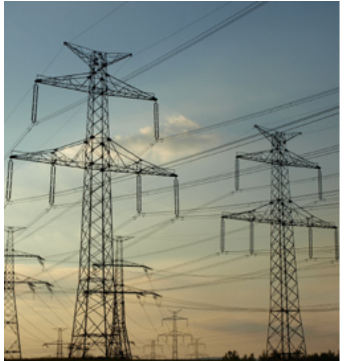
Electricity grids: assessing vulnerability, reliability and security of supply challenges
