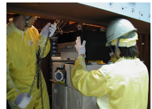
Layout of a specially designed neutron-coincidence counter (left) for Cm assay and its installation at Rokkasho (right).
