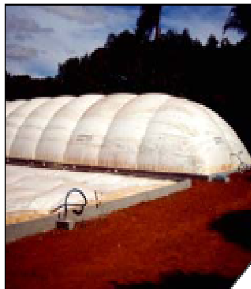
Project Activity Condition: Anaerobic Digester with Flare
